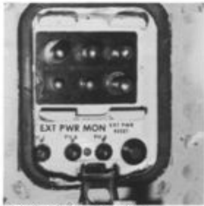
14 EXTERNAL ELECTRICAL POWER PANEL
